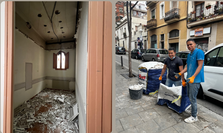
The first day of demo and hauling rubble to 'sacks'. No space for dumpsters on these narrow streets!
