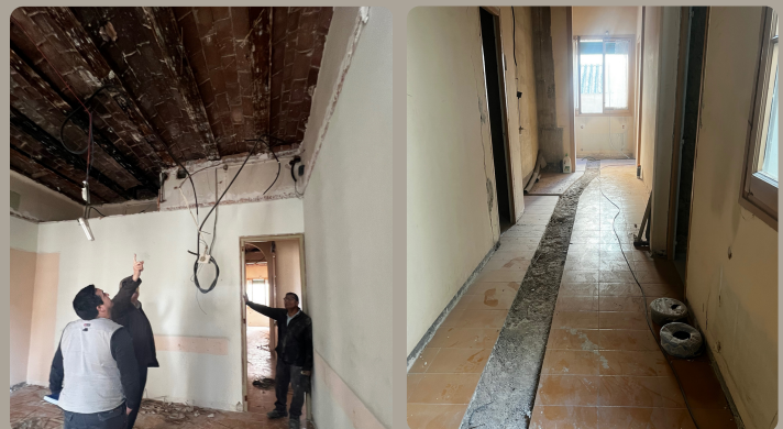
[L] Inspecting original ceilings and wooden beams [R] Trenches dug for water installations!
